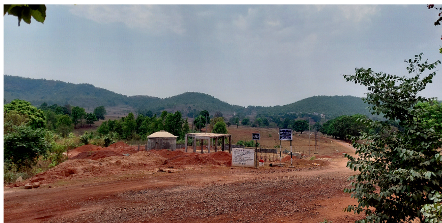
Fig. 2: View of the site Kusumita which is going to be destroyed as construction of water tank is in progress.
